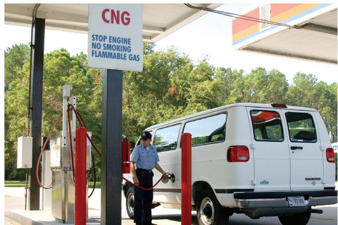
CNG Fueling Station (Image: U.S. Navy)
