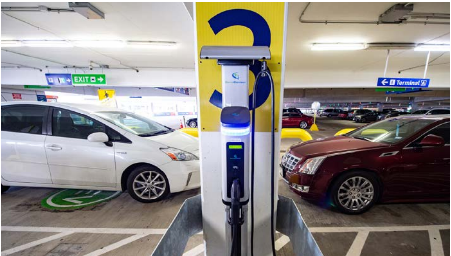
EV charging stations at Dallas Fort Worth International Airport.
